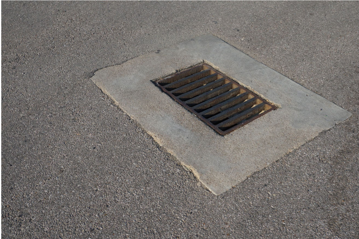
Photograph 6: Grated drainage inlets at subdivision entry roads and gas station entry
