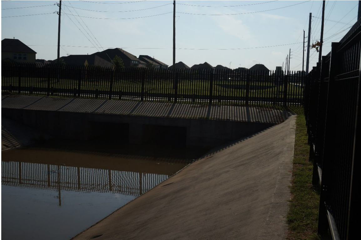
Photograph 2: Standing water in drainage containment Area (looking east)
