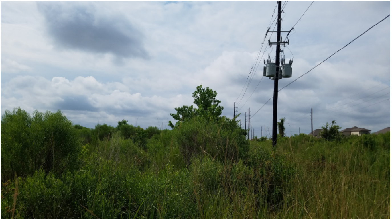
Proposed right of way on the east side of Porter Road – viewing south at SP1
