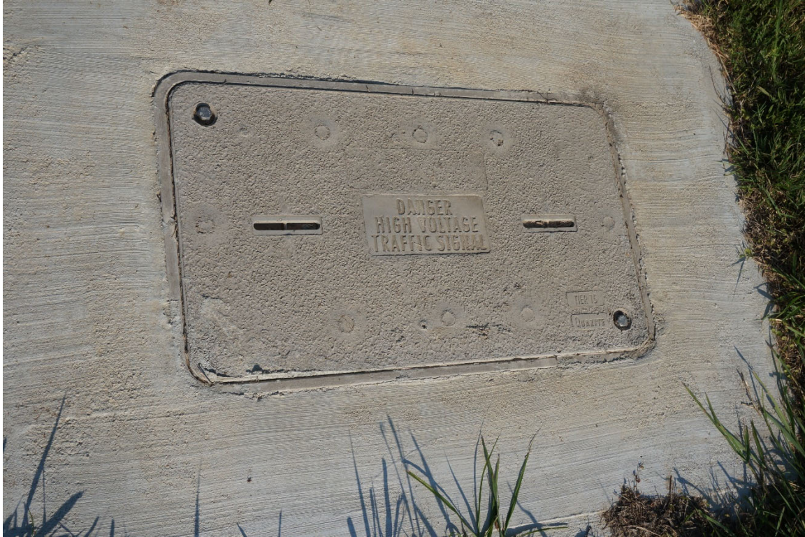
Photograph 5: High voltage traffic signal box cover (near intersection of Porter and Morton Ranch Roads)
