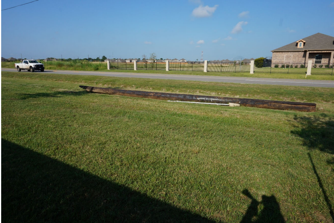
Photograph 17: Damaged creosote telephone pole alongside of Porter Road near Treviso Gardens Rd
