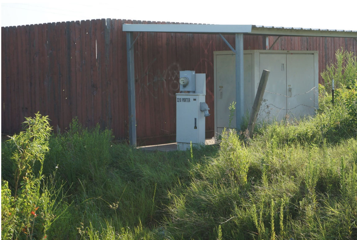
Photograph 14: Meter boxes near Water Treatment Plant
